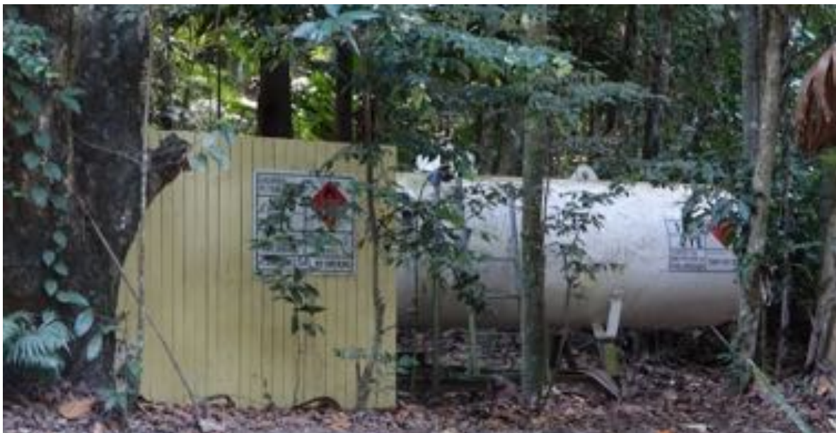
Fig 1.2 Large LPG Tanks, LPG used for Cooking and Heating (Primary Hot water), Typical Supplier Elgas
