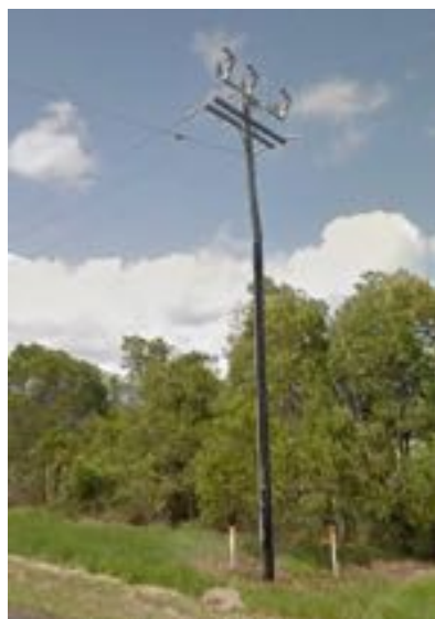
Fig 1.4 Typical Three Phase Ergon Hardwood Pole Structure Supplying Lower Daintree (with small conductor)
