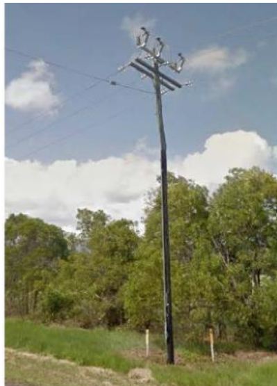
Fig 1.4 Typical Three Phase Ergon Hardwood Pole Structure Supplying Lower Daintree (with small conductor)
