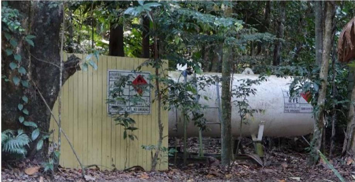
Fig 1.2 Large LPG Tanks, LPG used for Cooking and Heating (Primary Hot water), Typical Supplier Elgas
